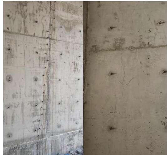
(b) Cracks in the basement shear wall of Jinmei Hainan City project
